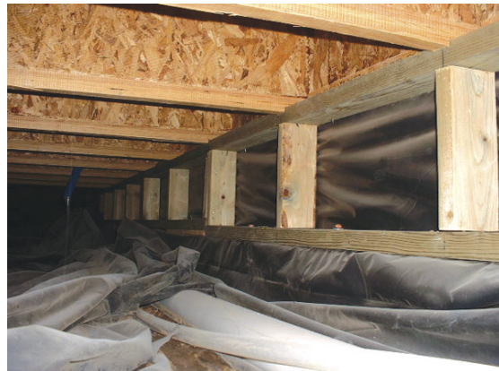
Figure SC-7: Conditioned crawlspace
