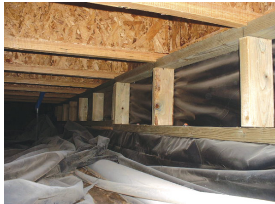
Figure SC-7: Conditioned crawlspace
