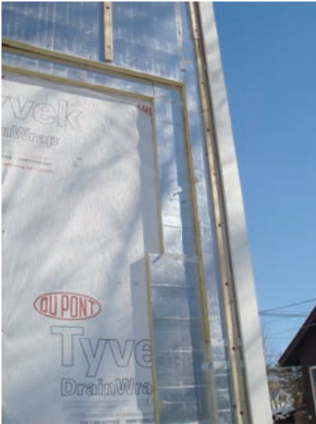
Photograph 7: Vapor Closed Foil Faced Continuous Exterior Insulation – Note the draining building wrap providing redistribution of moisture. And, yes, we were also here earlier...” BSI-071: Joni Mitchell, Water and Walls ”, November 2013).
