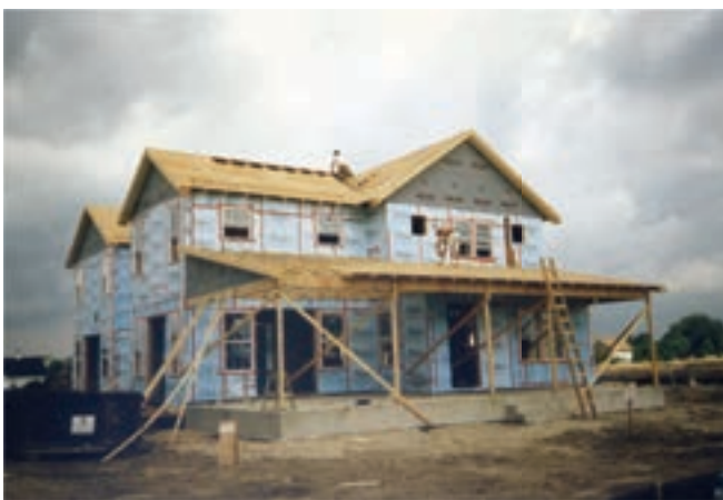
Photograph 4: Vapor Closed Exterior Continuous Insulation - If you used a vapor closed exterior continuous insulation like extruded polystyrene drying to the exterior was not possible.
