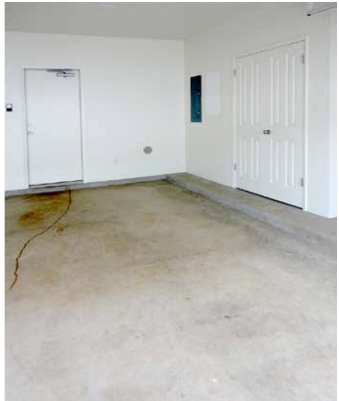
Photograph 3: Air Handler in Closet in Garage — Easy peasy right? Not if they are also gas furnaces. What about combustion air?
