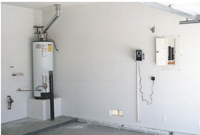
Photograph 6: Lonely Water Heater— Leaving the standard gas water heater outside of the closet solves the combustion air problem for the gas water in the closet as does changing the gas water heater for an electric water heater.
