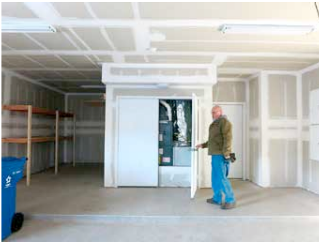
Photograph 5: Sealed Combustion— If the gas furnaces are sealed combustion and the water heaters are sealed combustion then transfer air from the garage is not necessary. Great approach...except... closet gets cold.
