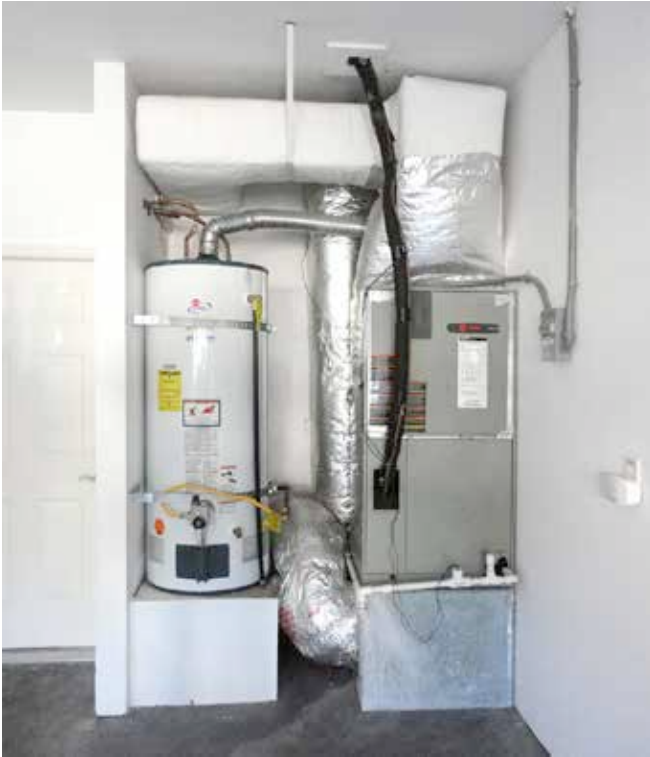
Photograph 2: Air Handler in Garages —There are complications. See Kevorkian. The air in an attic and garage comes from the same place...outside. Same dew point but higher relative humidity. It gets worse...wait for it...in a hot attic the box that makes air cold is actually warmer. Not so much in a garage. Air handlers themselves are colder as are the supply plenums that are attached to them. So stuff sweats more...way more. We actually increased moisture problems with equipment and ductwork when we moved air handlers from attics into garages.
